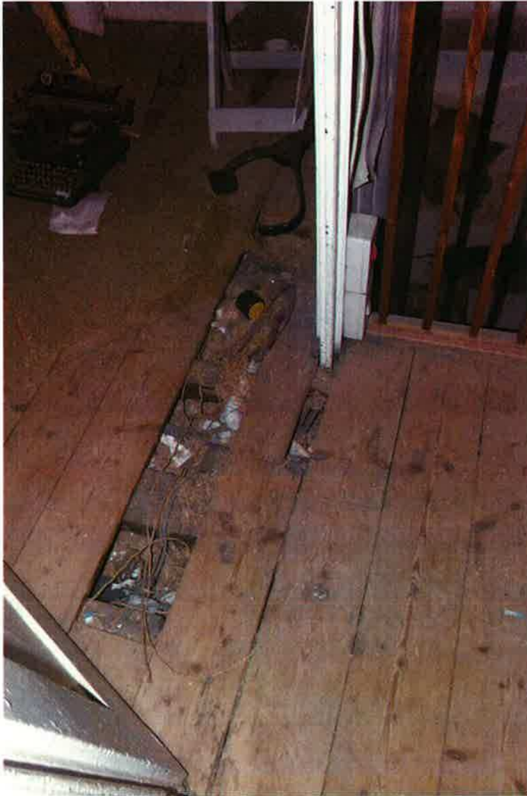
Many floor boards missing/removed – many rooms have been replaced with chip board
