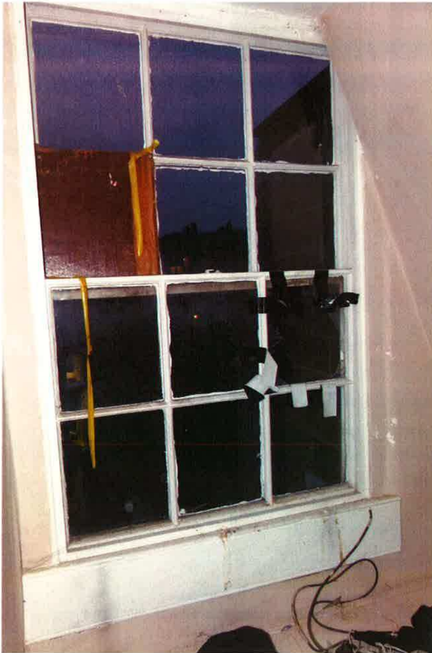
Typical condition of sash windows
