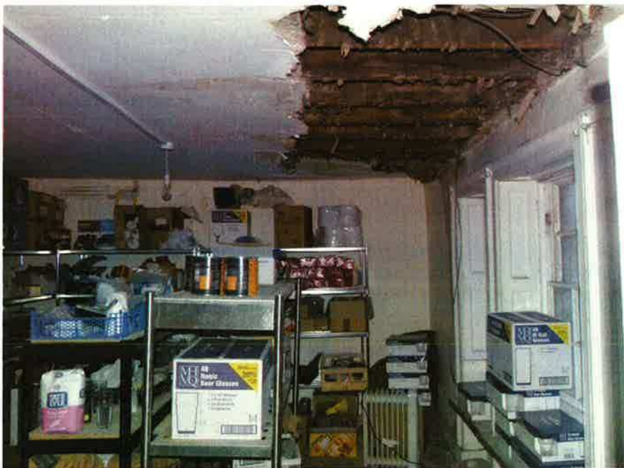
Room S6 – leak damage. Ceiling in danger of collapse
