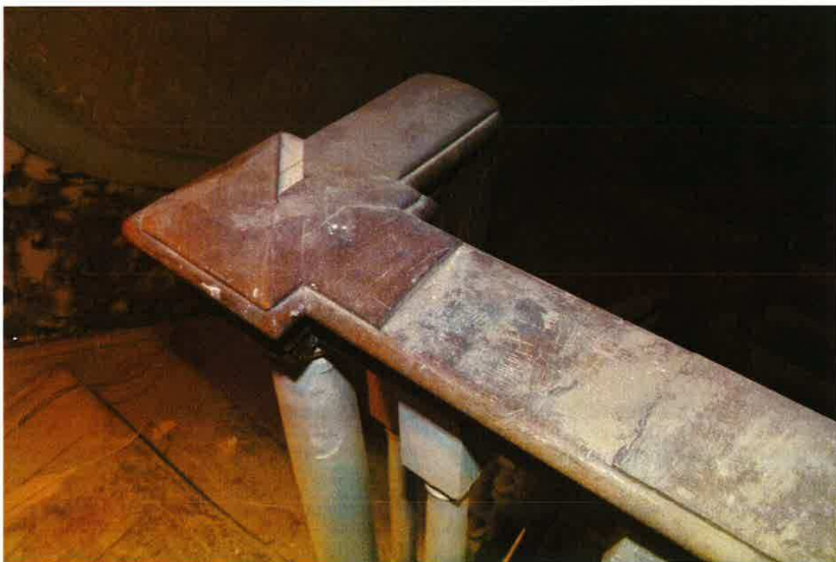
Banisters and Staircase in need of refurbishment
