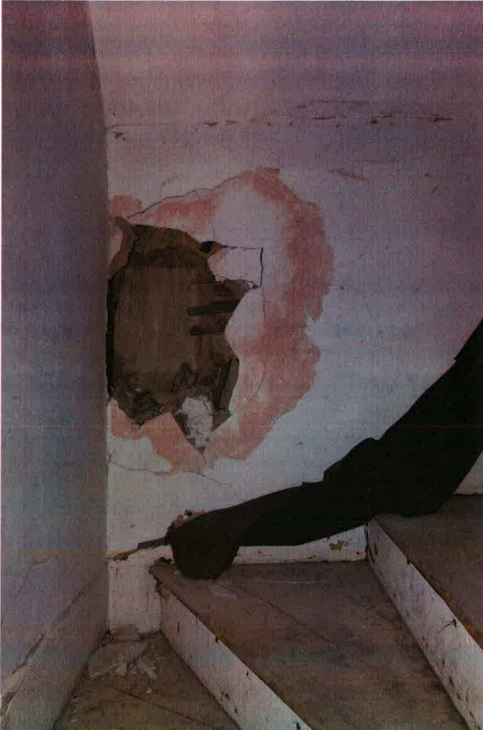
Plaster work in poor condition through building
