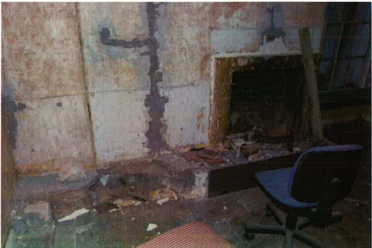
Rm S5 – derelict condition
